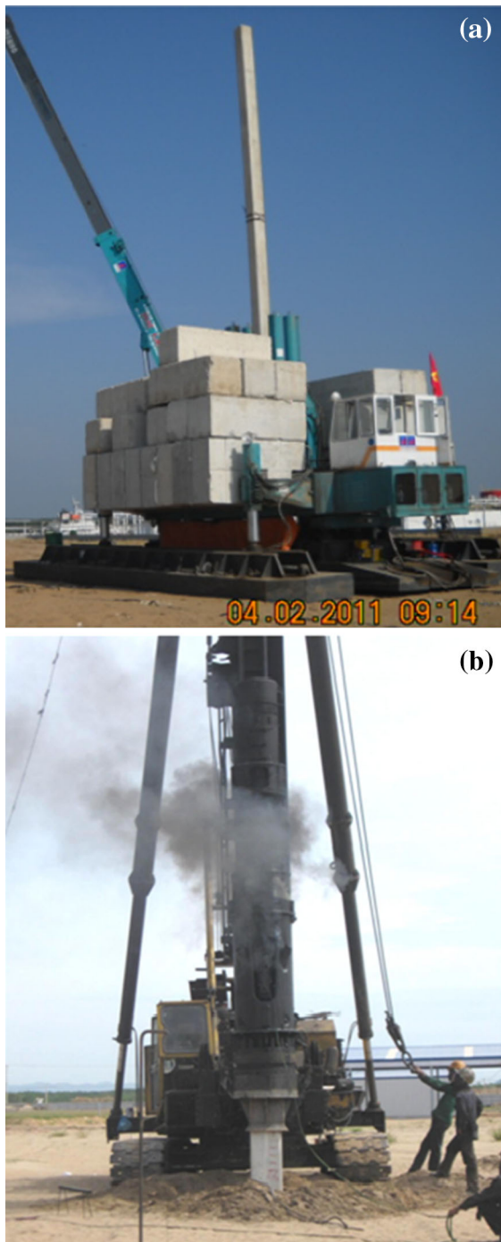
Fig. 8 a Hydraulic jacking system (Authors' photo). b Pile driving by KB45 diesel hammer (Authors' photo)
